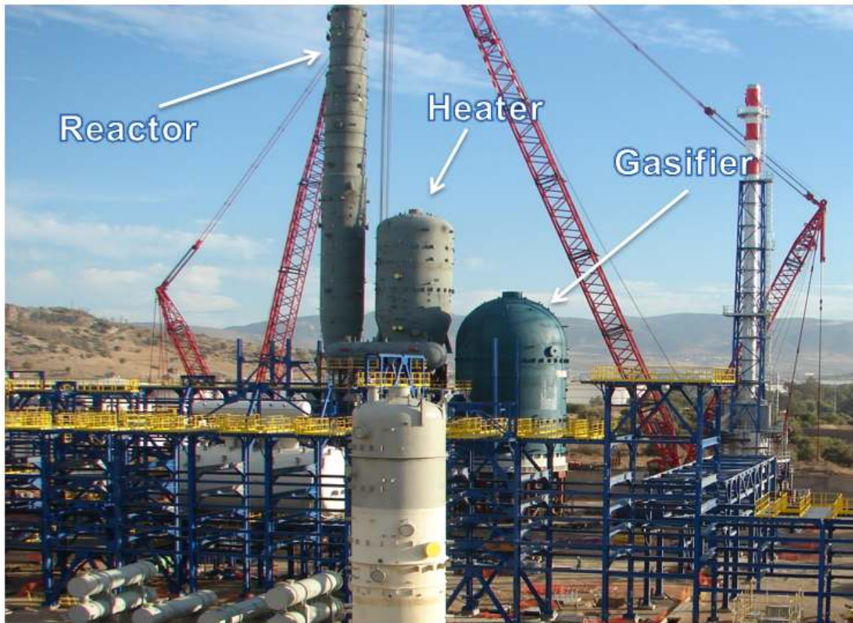
Figure 12. FLEXICOKING™ technology implemented at Hellenic plant
