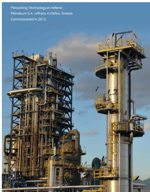
Figure 1. Unit at Hellenic Petroleum Elefsina Refinery
